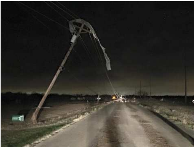
Utility poles, electric wires down on Hampton Rd. in Glenn Heights.
