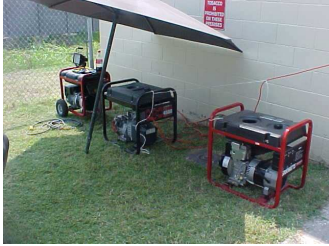
Portable power from generators
